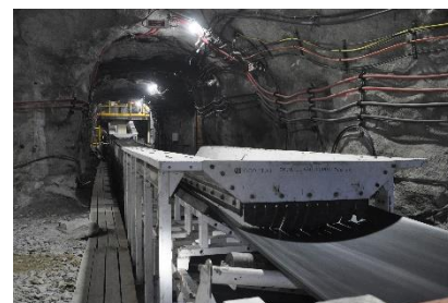
UNDERGROUND ELECTRIC CONVEYOR SYSTEM AT MAYSKOYE
