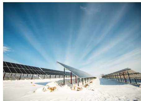
SOLAR POWER PLANT AT SVETLOYE
